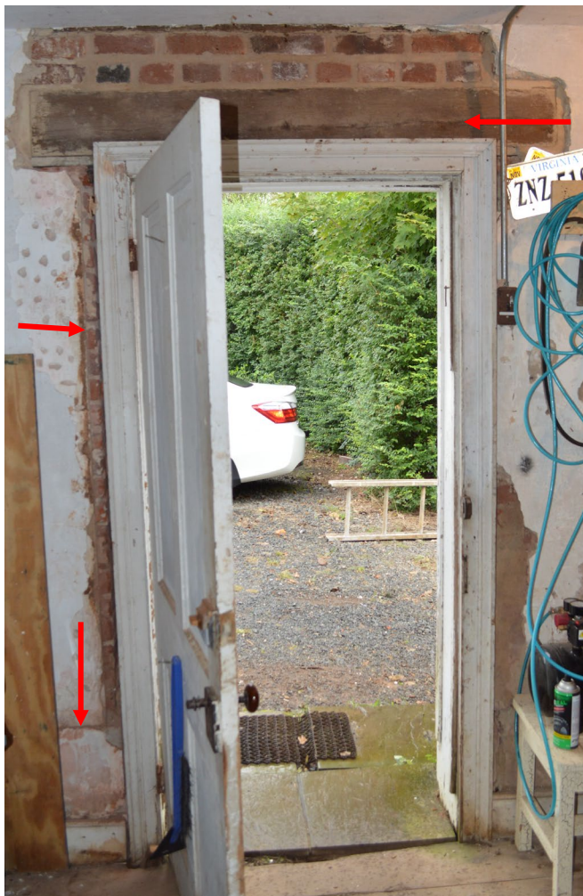
Figure 2. Room 101, northwest doorway (2018); replacement header, original door opening, and pre-ca. 1903 height of baseboard, all with red arrows.
