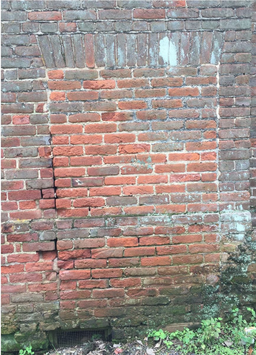
Figure 1. Pavilion north elevation, east doorway (2018); former entrance to cellar storage area, infilled.
