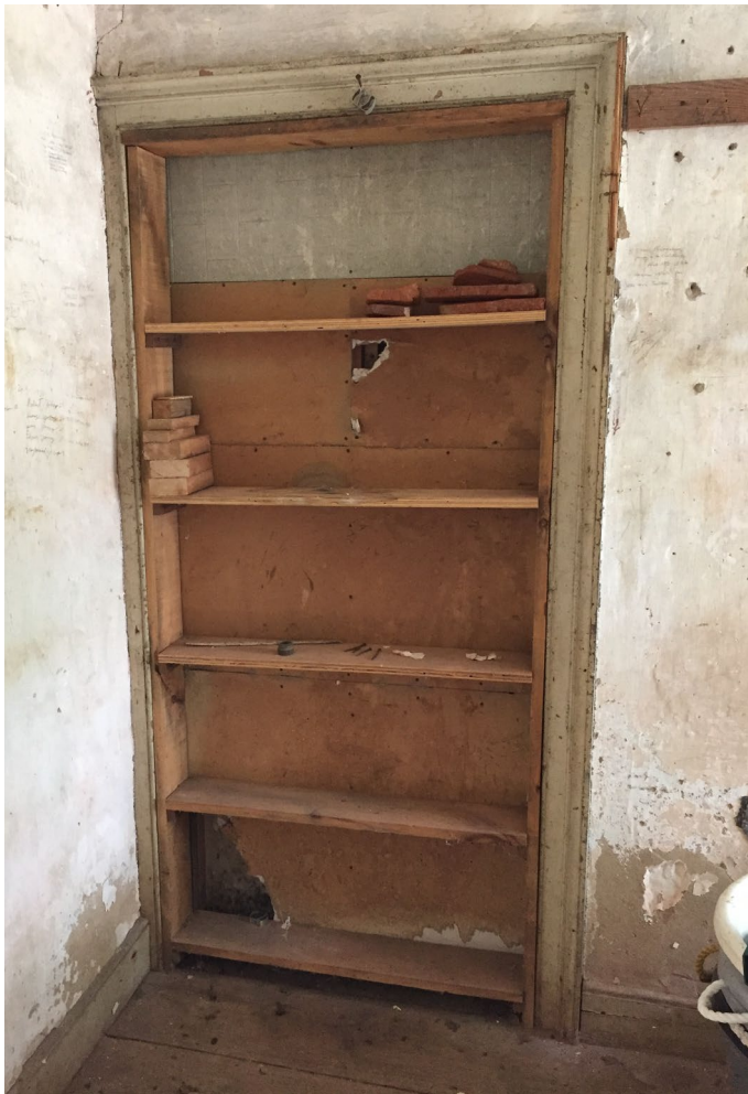
Figure 5. Room 107, blocked doorway connecting to Room 106 (2018); the opening and architrave are likely original.
