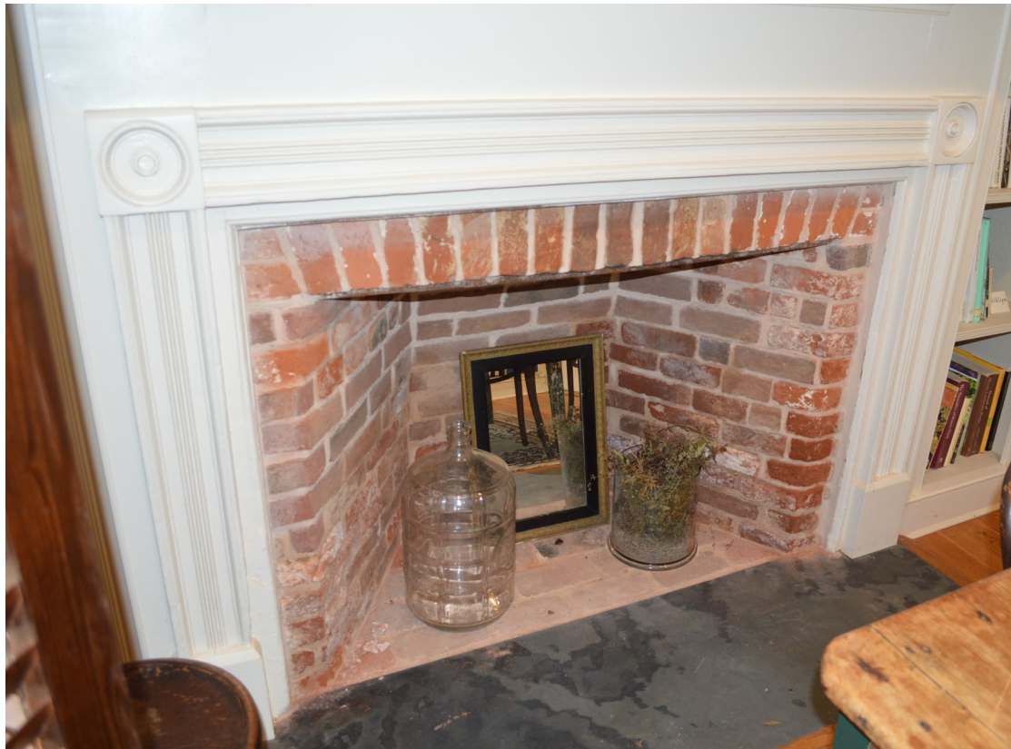
Figure 4. Room 103 fireplace (2018); while heavily reworked the overall size of the fireplace opening is likely to reflect the original condition.
