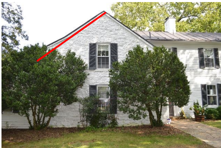
Figure 2. Little Oatlands Duplex 1, west elevation (2018); original pitch of roof indicated in red.
