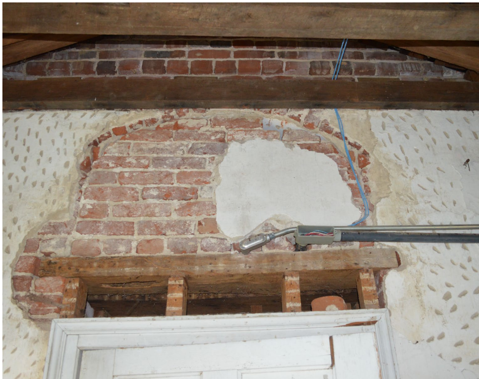
Figure 3. Room 102 with infilled former archway (2018); wood header and blocks to support brick archway infill; early plaster is just visible on the inner surface of the arch; ca. 1903 plaster with score marks to receive skim coat covers the walls and overlay the arch infill.
