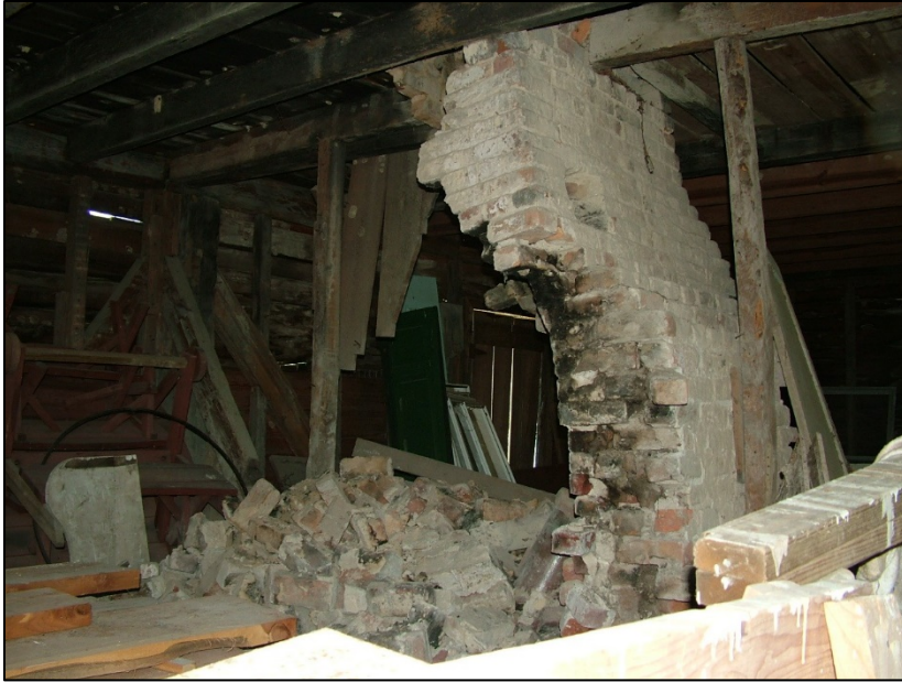
Figure 4. The central fireplace mass and chimney in the Four Square quarter has almost completely fallen, and the entire structure is in imminent danger of collapse.
