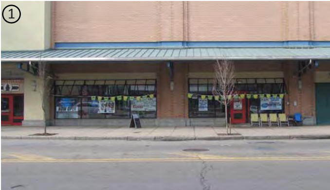
① Stretching along Lackawanna Avenue are a series of overhangs that direct stormwater into the building through gutters.
