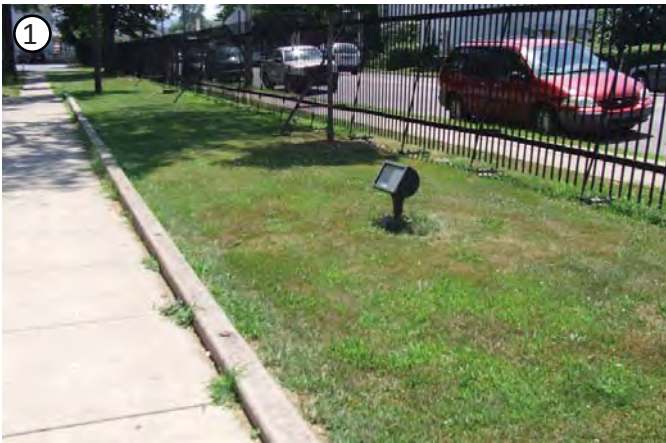
Currently water hits the curb of the sidewalk and runs down it until entering the street.
