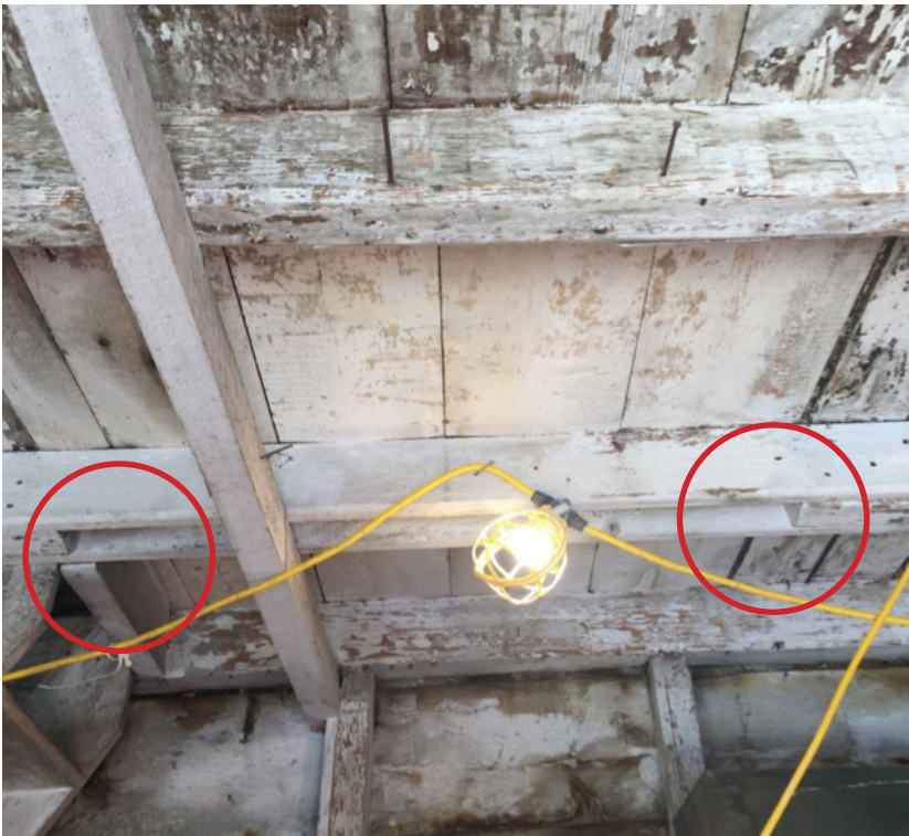
Figure 8. Detail of the frame along the north wall, east of the stairway, and the patch in the ceiling floor; the ends of the short joists are sistered with 1" planks (circled in red) (2018).
