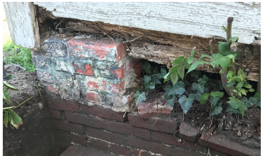
Figure 4. Southwest corner of the Bayly outbuilding, with the current pier resting on an earlier pier or partial foundation (2018).
