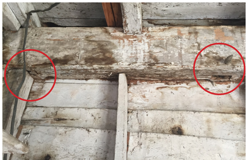
Figure 7. East wall frame detail, with original girt (chamfered corners) and two mortises in the bottom face, for the original corner post (left) and the door post (right); the narrow stud was inserted after the doorway was relocated (2018).
