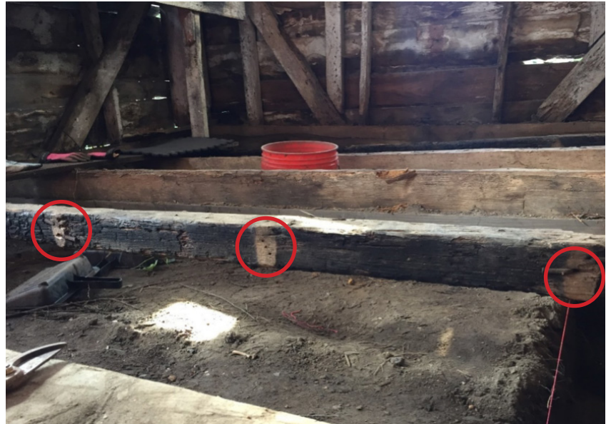
Figure 15. Facing west, replacement floor joists; with two reused joists each with three charred faces, ghost marks for studs, and protruding cut nails (2018).
