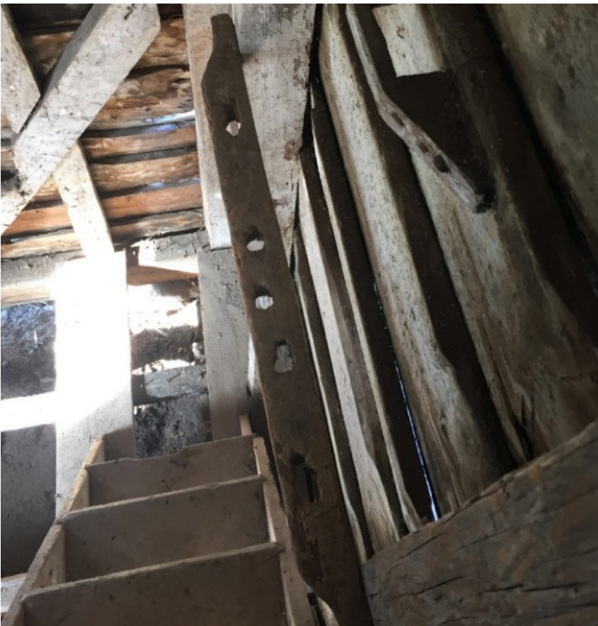
Figure 14. Detail northwest corner interior, with wood tool rack attached to two wall studs and a wood handle attached to the back of the weatherboard siding (2018).
