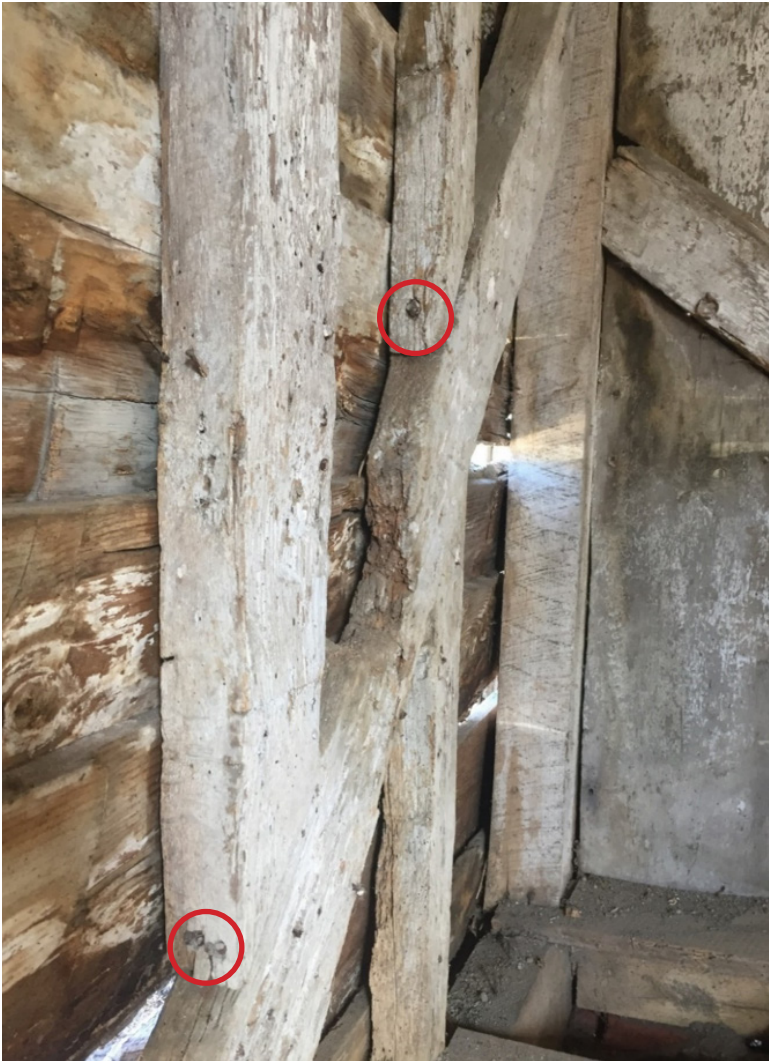
Figure 5. Northwest corner interior, showing the replacement corner post and sills (circular sawn), and two original down braces and two studs; studs are attached to the braces with wrought nails (2018).
