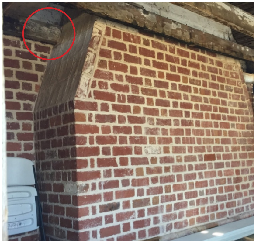
Figure 9. The exterior of the chimney base of the Machipongo kitchen, incorporated within a 19C addition; in this instance, the end joists of the addition were cut on an angle to rest against the sloping shoulder of the earlier chimney base (2019).
