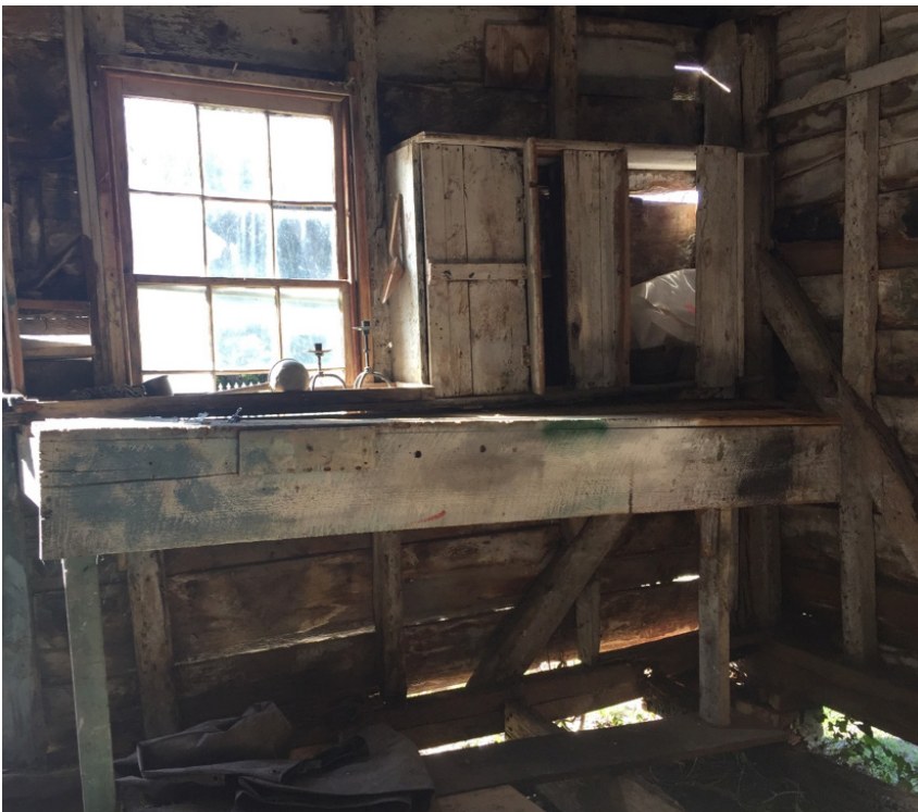
Figure 12. South wall interior, west of the doorway (P2), with cabinet and counter (P3), work bench and window (P4); southwest corner post and braces are original (2018).
