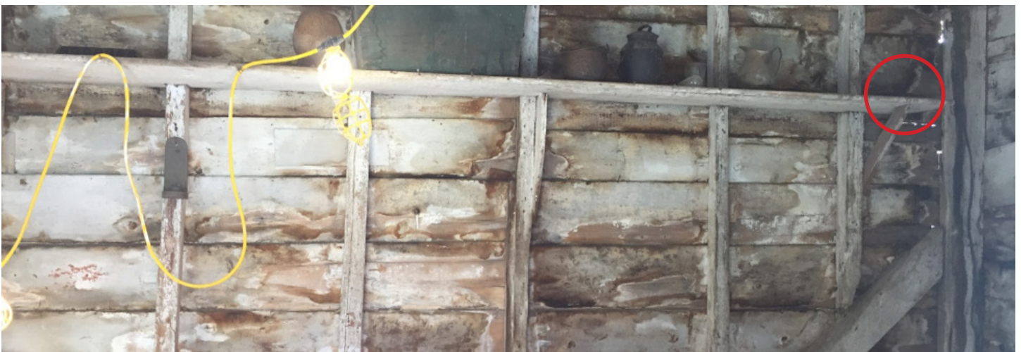
Figure 11. The north wall interior of the Bayly outbuilding, showing original plate, studs, and northeast corner brace, and replaced post, sill, and joists; the end of the shelf is beveled to overlap the shelf board that ran along the east wall; end of shelf and inserted bracket circled in red (2018).
