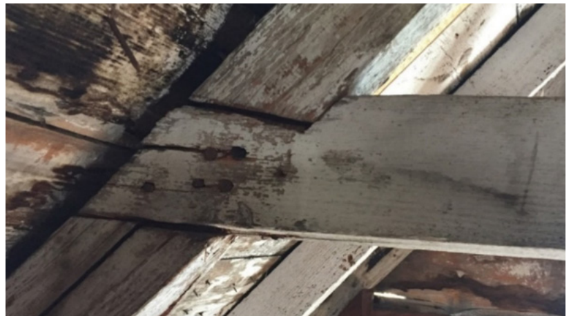
Figure 6. The roof frame has been substantially altered. One collar appears to be in its original location, attached to the rafters with a half-dovetail joint, and fastened with both cut and wire nails (2018).
