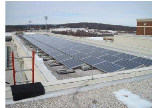
Frederick County Oakdale High School – Ballasted Rooftop Mount
