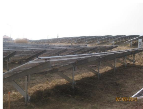
Back River WWTP – Screw-type Ground Mount
