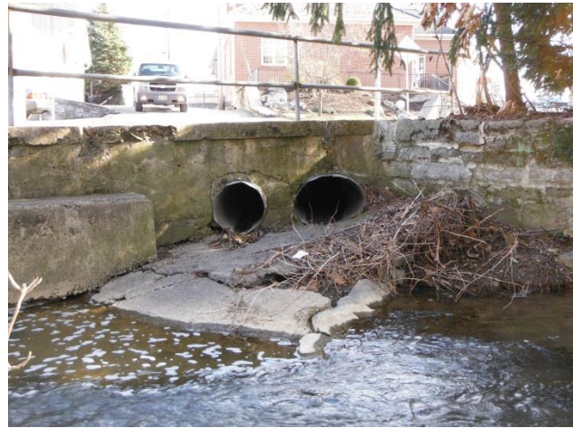
Figure 3 – Example stormwater outfall located at N. Park Ave with direct untreated stormwater connection to Johnston Run.
