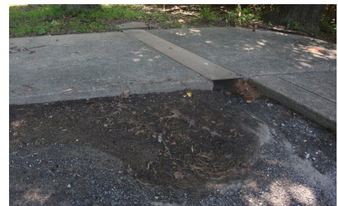
Figure 19 Drain debris lot 311
