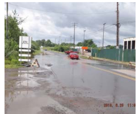
Flooding along Boulevard Ave. near I-81 swale
