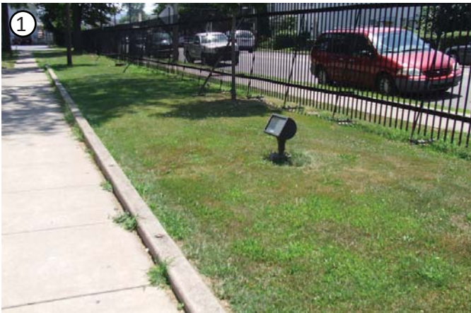
1 Currently water hits the curb of the sidewalk and runs down it until entering the street.
