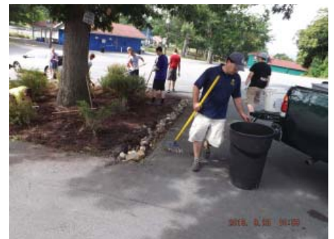
Constructing a bioretention area at Nay Aug Park with University of Scranton volunteers.
