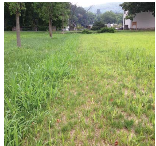
Hillside Farms in Shavertown, PA used a grid system filled with grass for an overflow parking area instead of traditional asphalt. The grass fits in with the farm atmosphere. (Picture above is 1st year of growth.)
