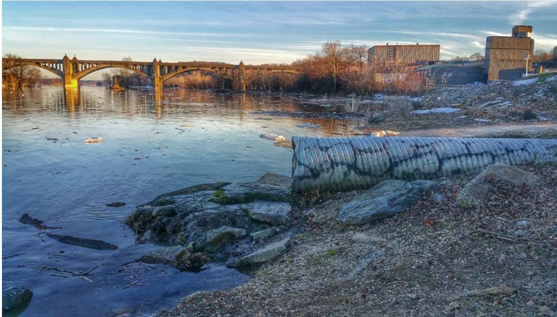
This photo highlights the importance of maintaining Wrightsville's stormwater infrastructure which flows directly into the Susquehanna River; Photo credit – E. Reed
